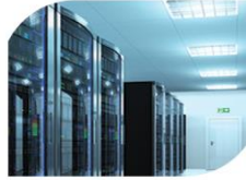
DATA CENTRE FUEL TESTING
